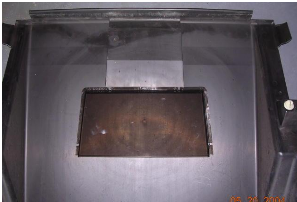
Figure 17: Wall pocket on radiator cover
